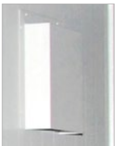
Air vents with fire protection
