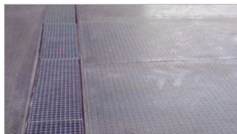
Gutter with grid
