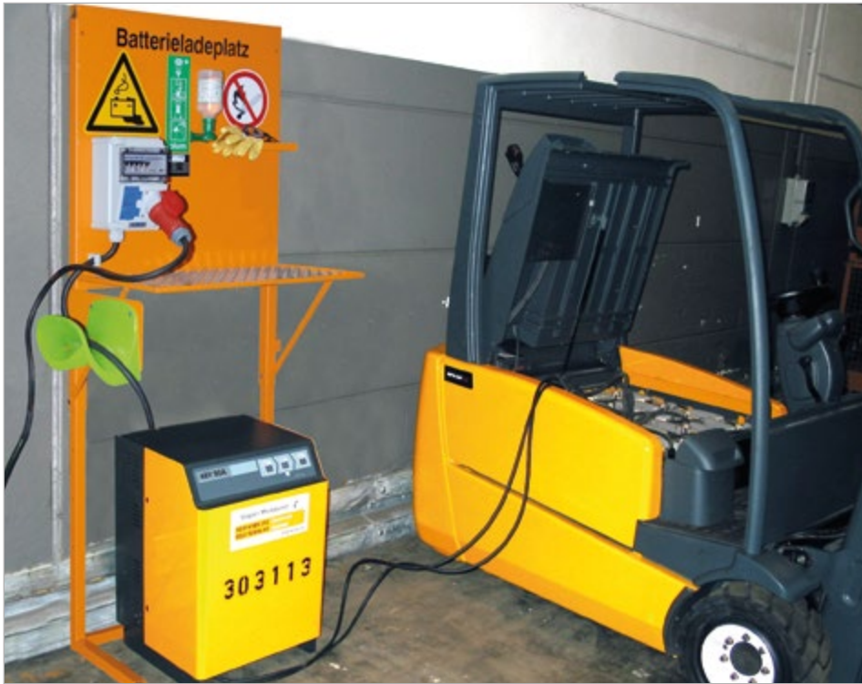
Type BL with fire extinguisher, with CEEform socket 400 V charging the battery of an electric forklift truck
