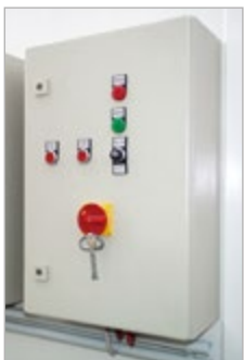
switch cabinet with control keys
