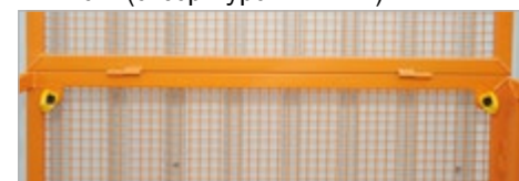
anchorage points for protective equipment
