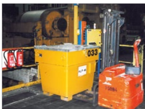
Mobile oil supply for machines
