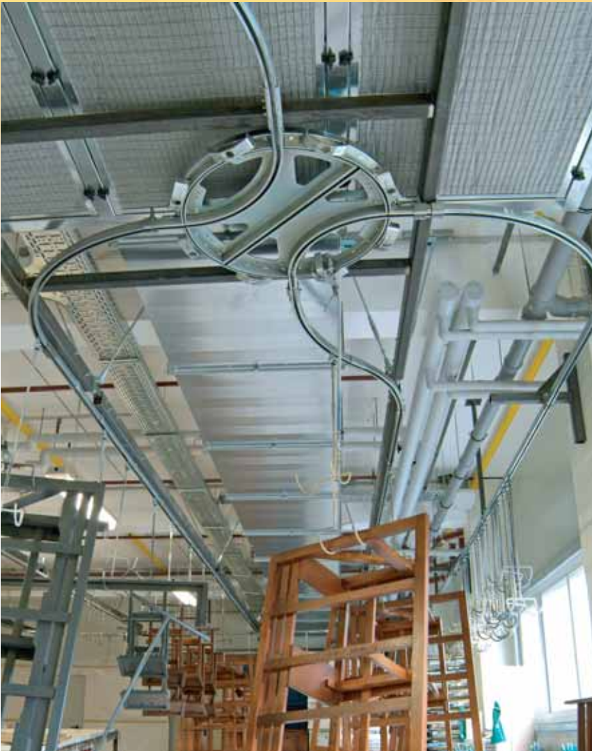
Overhead conveyor system with Müsing spider assembly.
