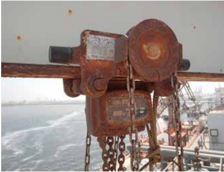
Corroded Yalelift with integrated trolley – still functional after 9 years in use
