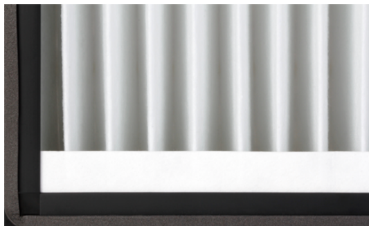
Water barrier and gasket on the downstream side
